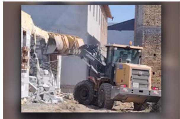
The demolition of a Council of Churches Baptist building. Photo: Baptist Council of Churches
